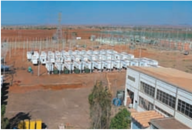
The 170 MW emergency power plant in Zacatecas, Mexico, used the large Cummins Power Generation North American Rental Power fleet.
